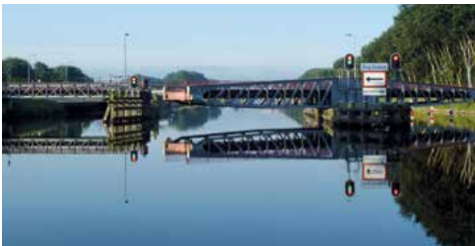
This heritage swing-bridge in Souburg was refurbished and fitted with InfraCore® Inside decks.
