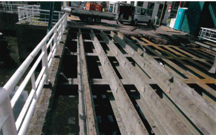
Deck refurbishment: the original timber deck has caused the supporting steel structure to be in bad condition.
