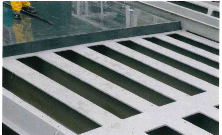
The steel structure has been repaired and conserved, followed by the installation of the first InfraCore® Inside deck segment.
