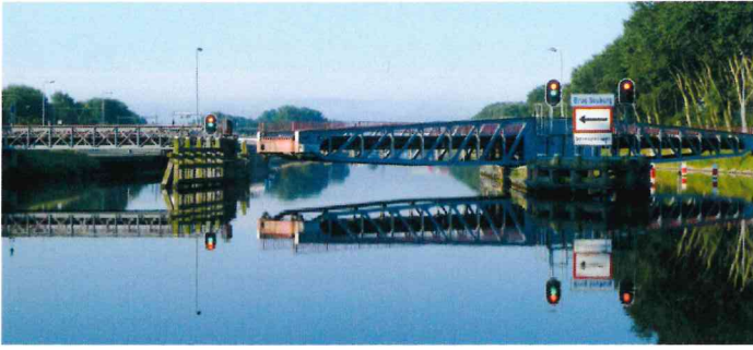
This heritage swing-bridge in Souburg was refurbished and fitted with InfraCore® Inside decks.
